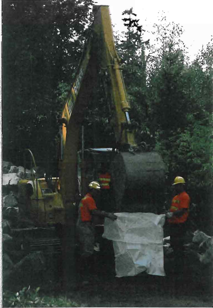
Boulders were bagged at the staging area and then airlifted to the project site. PACE Engineers/SWSSD
