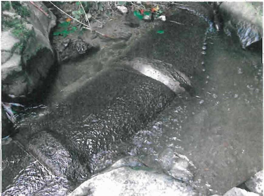
District staff discovered that sewer lines and several manholes, which previously were buried beneath the stream, had been exposed. PACE Engineers/SWSSD
