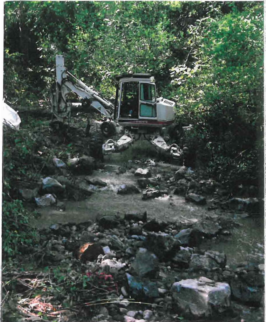
The Spyder Hoe excavator was chosen for its ability to "walk" up the creek channel with minimal environmental disruption. PACE Engineers/SWSSD
