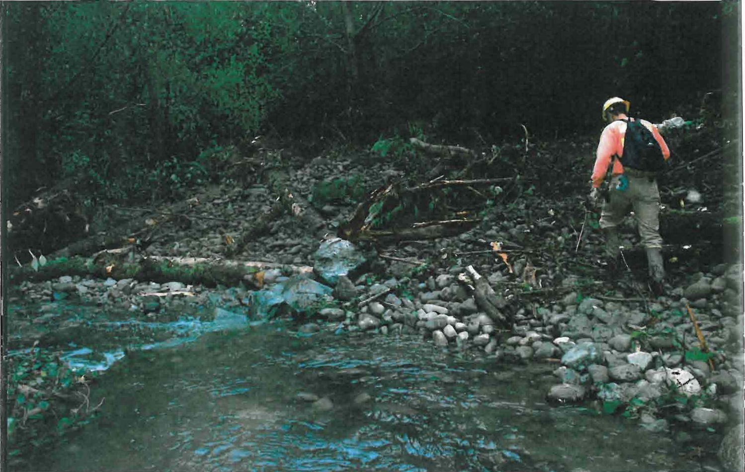
Post-construction, the stream channel has been raised to its 1966 conditions and constructed to minimize future erosion. PACE Engineers/SWSSD
